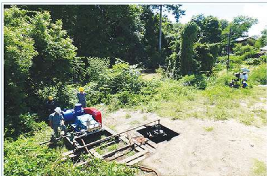
Fig. 05: Injecting Produced Water to M 132
